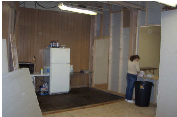
Business end of service area, to become kitchen. The fridge is the location of the future bathroom.
